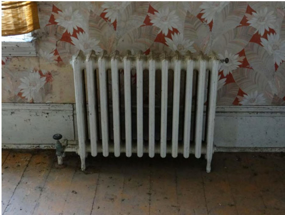
Plate 42: Cast iron radiator in living room two.
