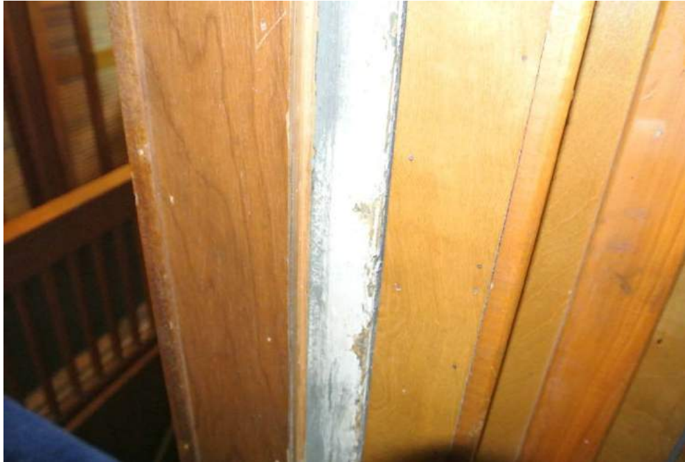
Plate 35: Detail of the former exterior west wall of the original structure, now creating the boundary between the original residence and the modern addition.
