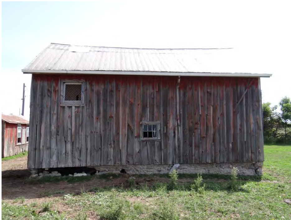
Plate 108: West elevation of the piggery (P). Note the crumbling foundation at the lower left base.
