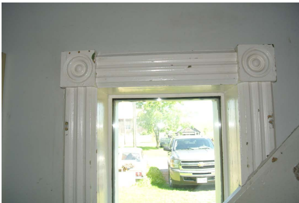
Plate 32: Detail of partially obstructed original window on the north wall, next to the stairs.
