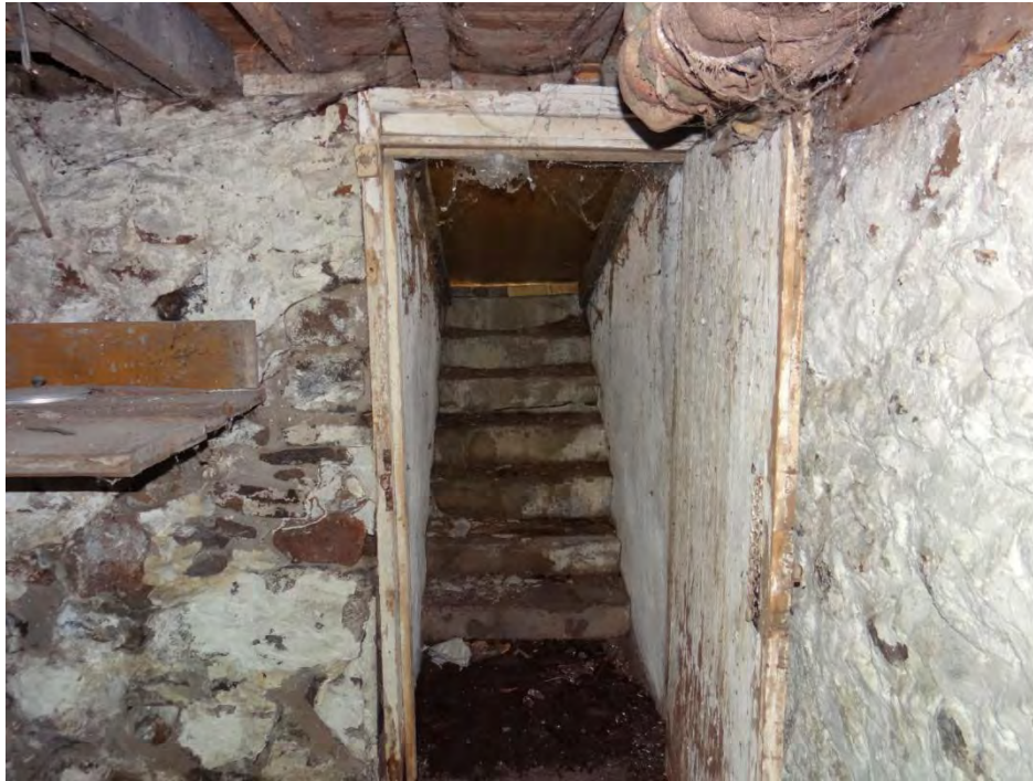
Plate 84: Photo of the basement stairs that lead to the exterior storm door on the south elevation.
