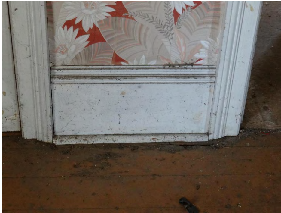
Plate 43: Detail of moulded baseboards in living room two. These baseboards are likely original.
