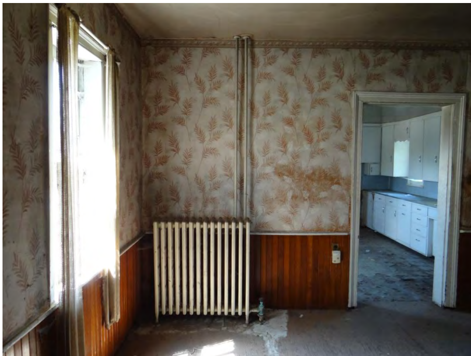
Plate 37: Cast iron radiator in living room one. The kitchen is visible through the door on the right.
