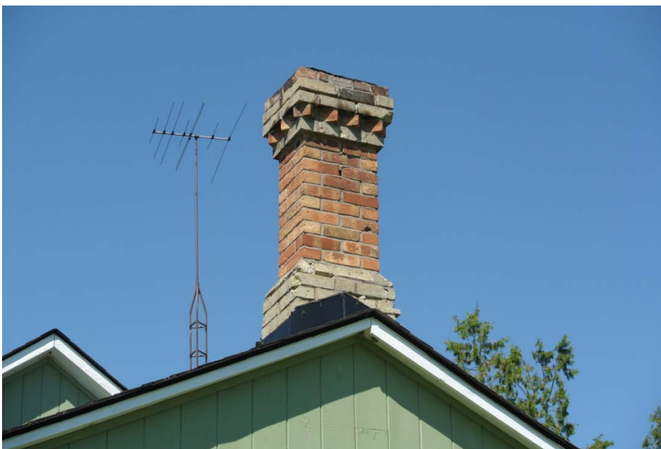
Plate 8: Brick chimney stack on east elevation of the original portion of the house. Note the elaborately corbelled top and combination of buff and red brick.
