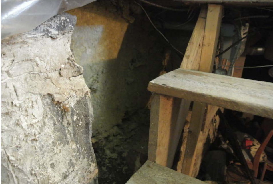
Plate 49: Detail of gap in the foundations on the north wall.
