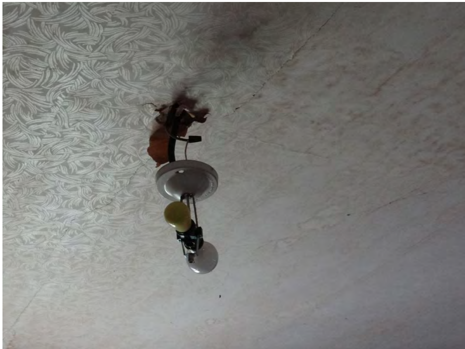
Plate 46: Photo of overhead light fixture in living room two.
