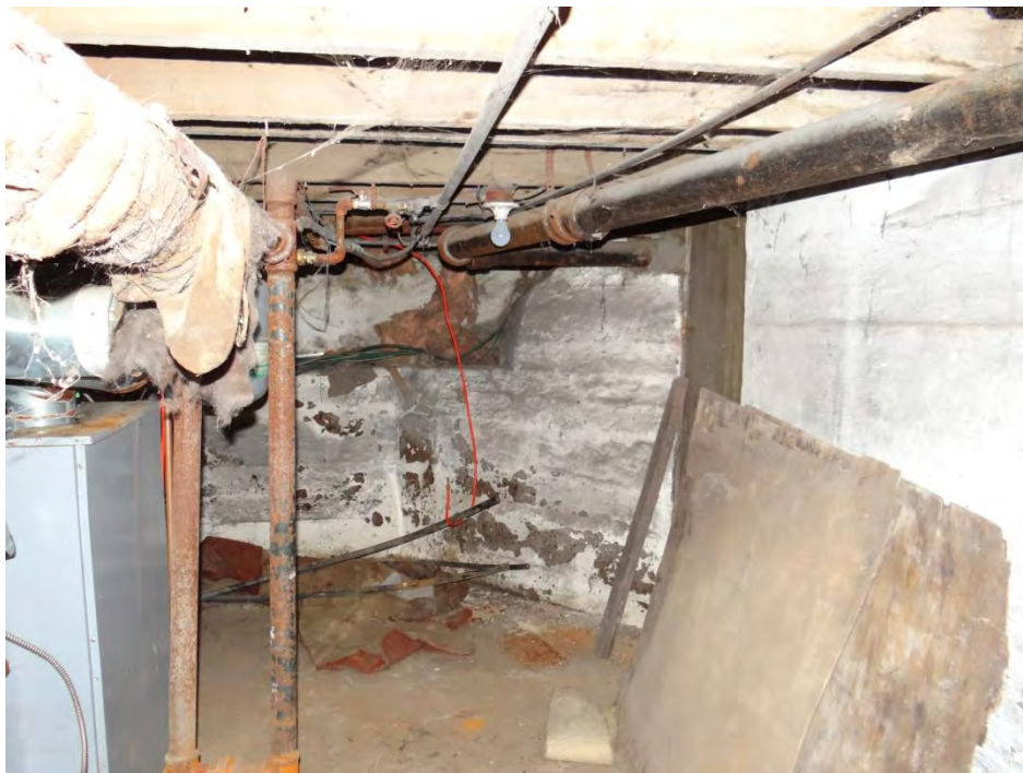
Plate 89: Photo of the basement under the north section of the house. Note the parged walls, dirt floor, and home heating/electrical systems.
