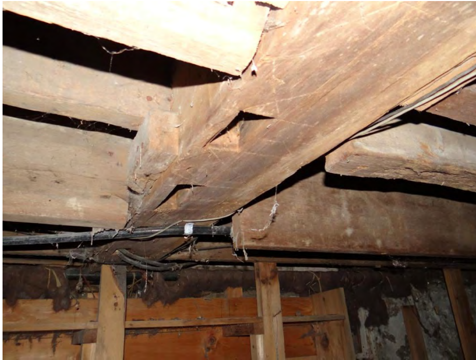
Plate 86: The summer beam in the basement (original south section). Note that the summer beam is hand hewn but that some of the cross beams appear to be newer/replaced.
