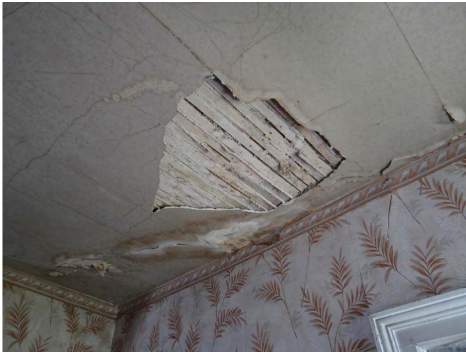
Plate 39: Exposed lath and plaster construction in living room one.
