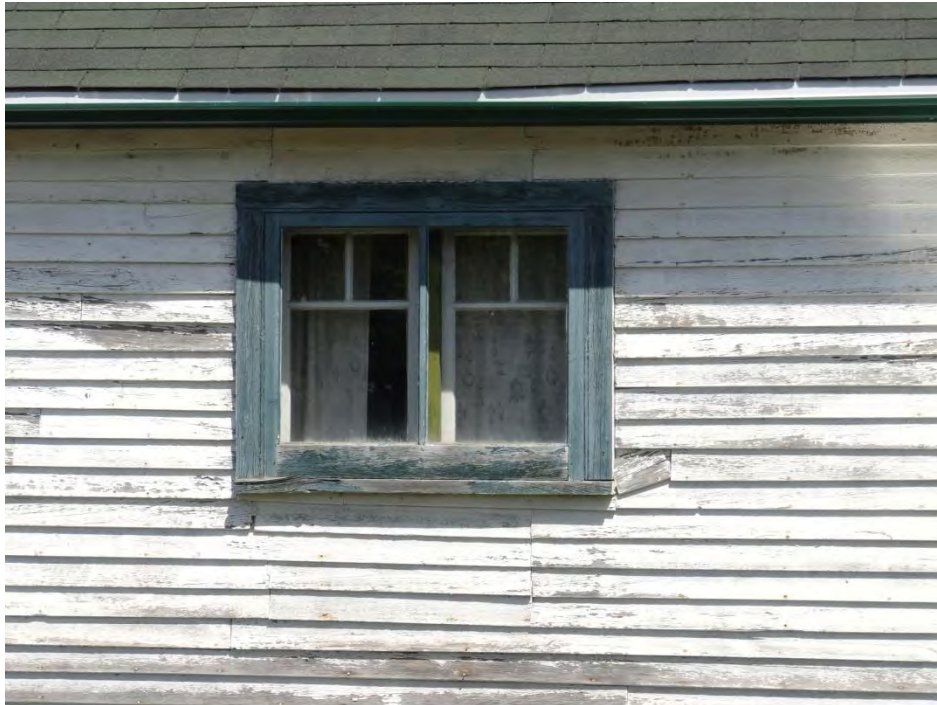
Plate 29: Example of a two-over one casement window located in the kitchen tail (south elevation).
