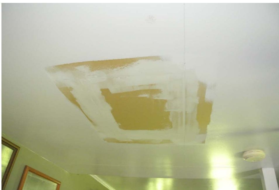
Plate 24: Detail showing patchwork from a former leakage problem.
