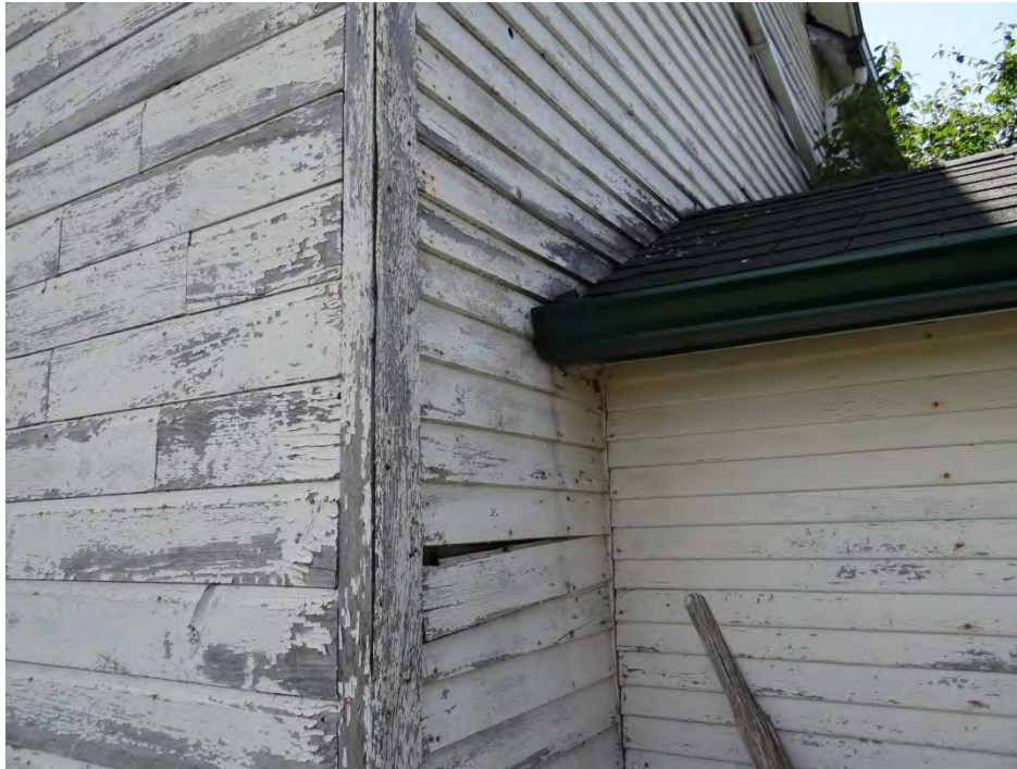
Plate 7: Photo showing shiplap siding on the north elevation and clapboard siding on the west elevation.
