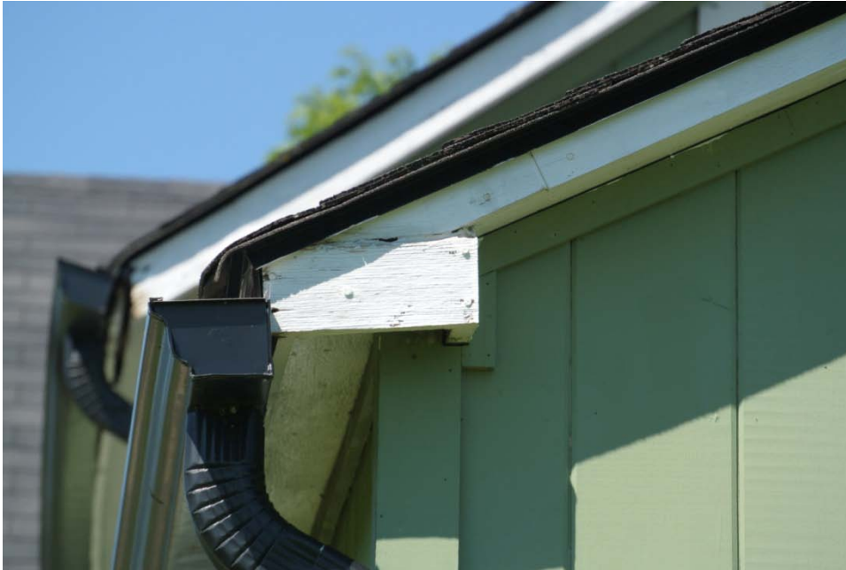
Plate 7: Detail of vertical wooden clapboarding and wooden fascia, soffit and return eaves.
