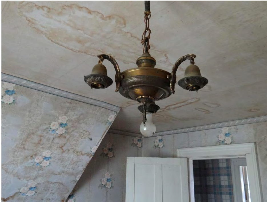
Plate 70: The brass overhead light fixture in bedroom two.
