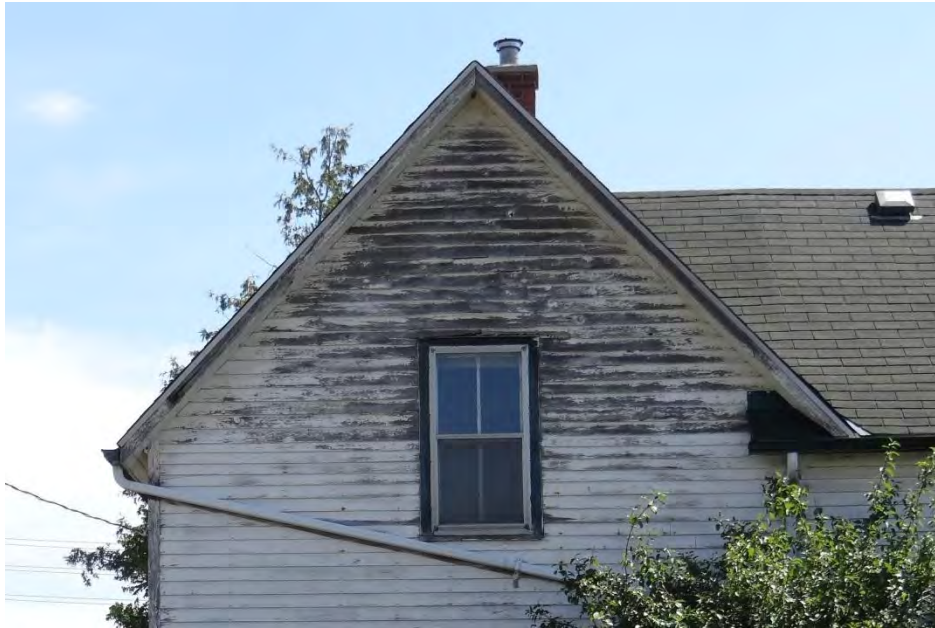
Plate 11: Photo of the gable roof on the north section of the residence (west elevation).
