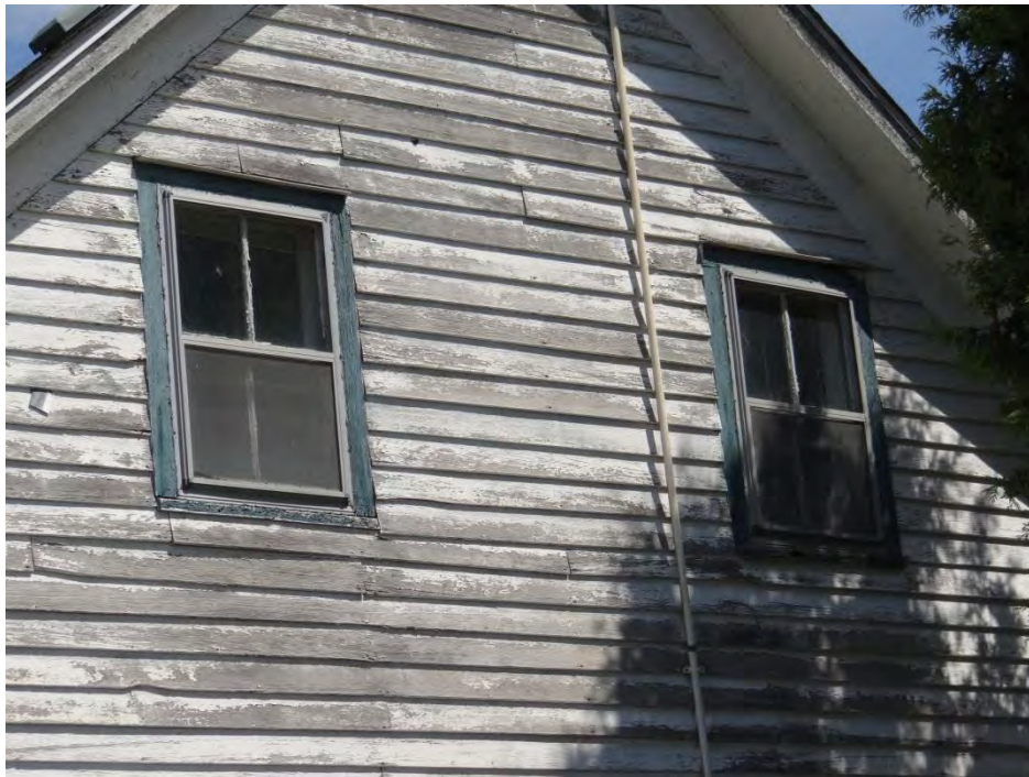
Plate 26: Two-over-two sash windows located in the original south section of the house (south elevation). The original wood storm covers have been replaced with aluminum frame covers.
