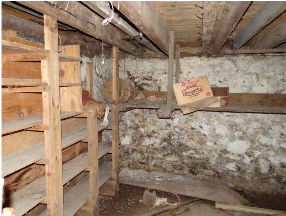
Plate 85: The basement under the original south section of the house. Note the stone foundations, dirt floor, and relatively new/replaced subfloor.
