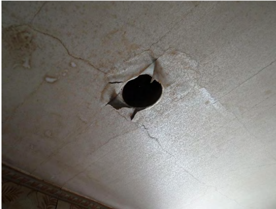
Plate 38: Photo of a vent or possible wood stove chimney hole in the ceiling of living room one.
