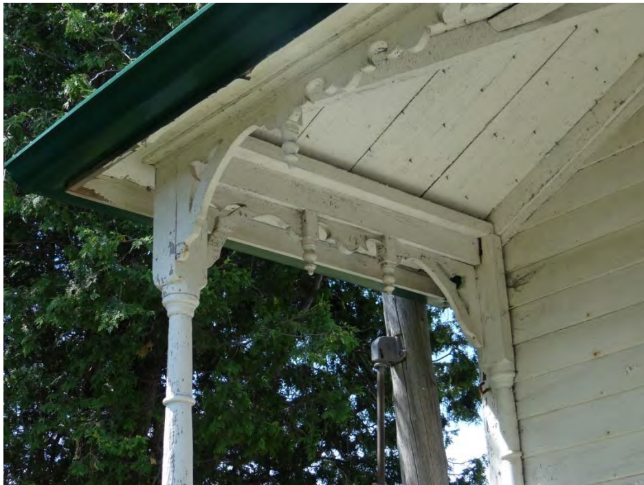
Plate 30: Photo of the turned columns and decorative vergeboard located on the front façade (east elevation).
