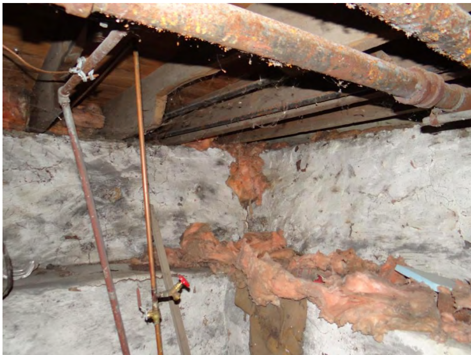
Plate 91: Photo of the beams in the north section of the basement. The beams here are sawn.
